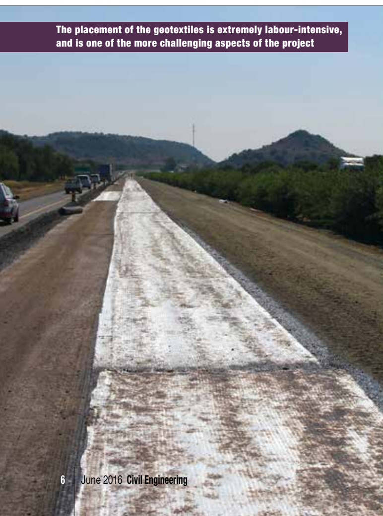
Accurate spreading is done by hand, meeting SANRAL's labour requirements, and then compacted mechanically
